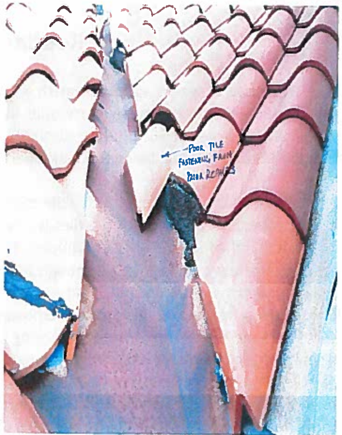
Figure 2 Poor tile fastening from prior repairs
